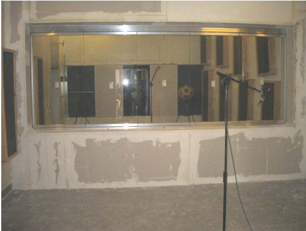
Fig. 1: View Transmission Room, Measurement 1
